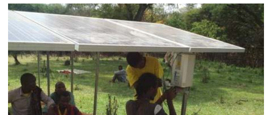
Gobile village water supply scheme equipped with solar powered submersible pump
