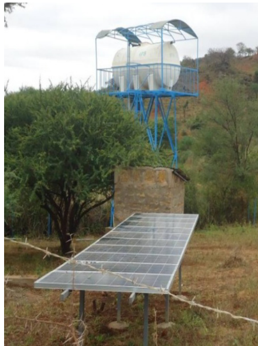
Water supply scheme equipped with solar powered submersible pump
