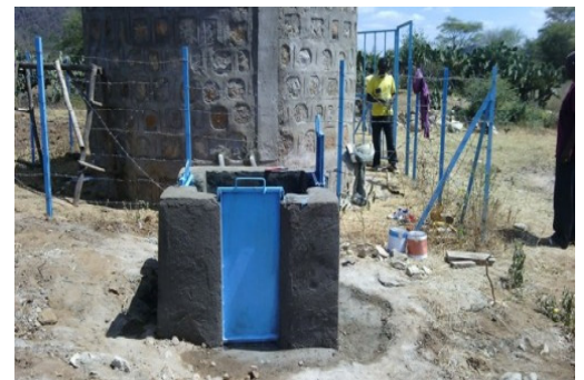
Water collection and division chamber for small scale irrigation scheme
